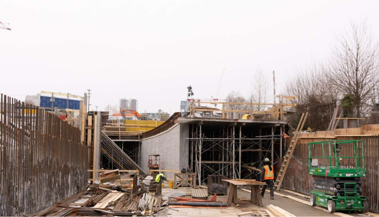
Figure 2: Great Northern Way-Emily Carr Station: Progressing with construction of the transition box tunnels.
