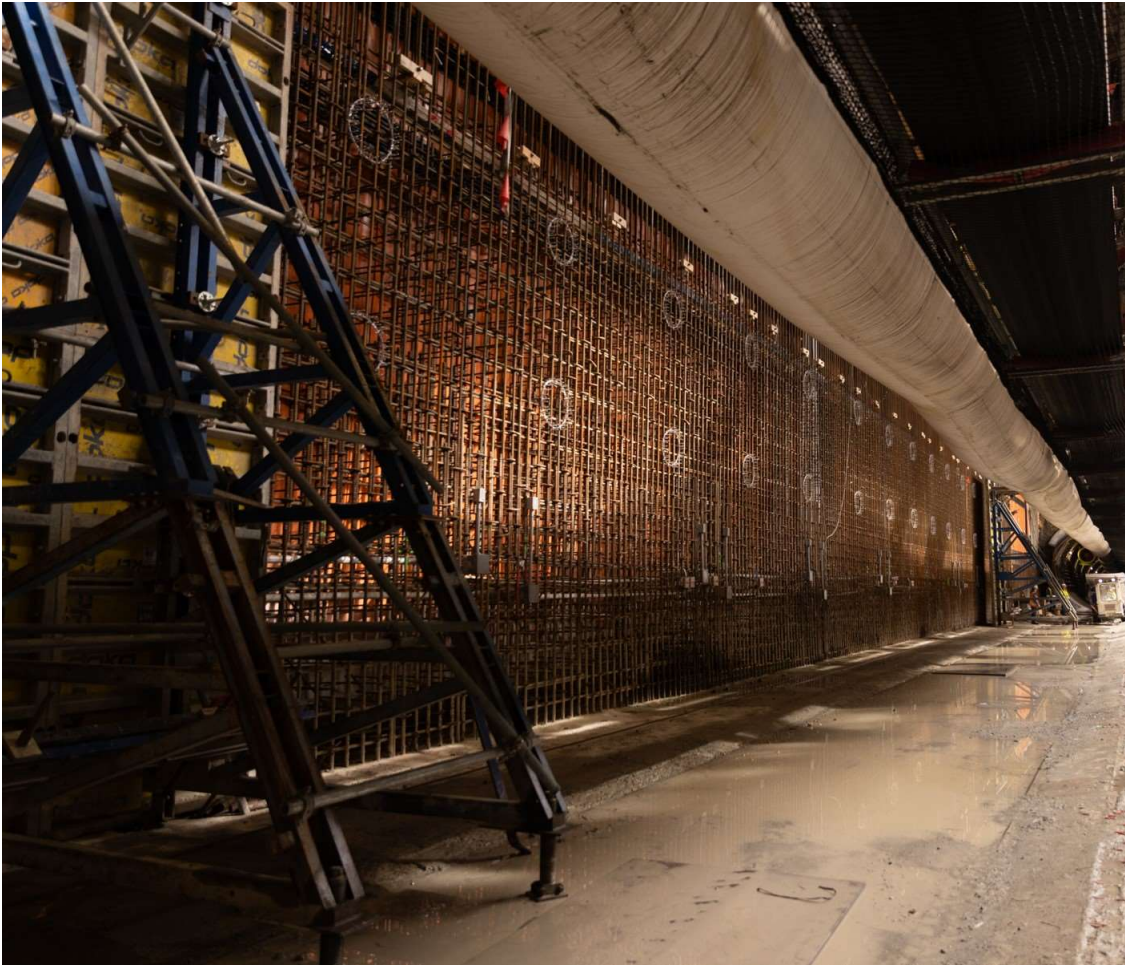
Figure 5: Oak-VGH Station: Progressing with rebar installation and concrete pours for the station box exterior walls.
