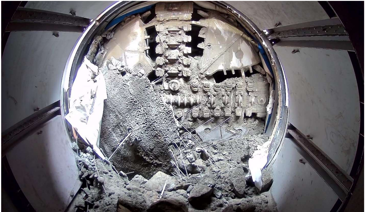
Figure 7: Arbutus Station: Arrival of TBM Phyllis into the specialized pressure chamber on March 20.
