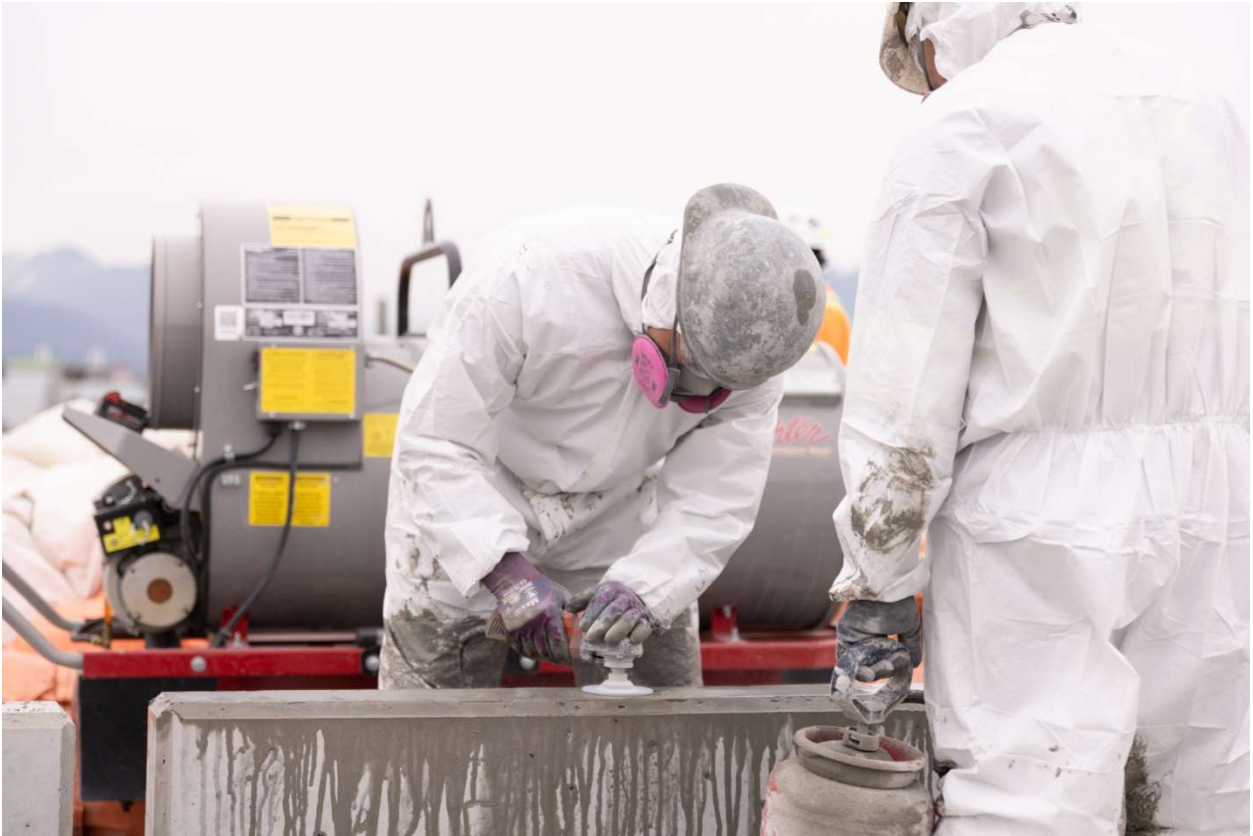
Figure 1: Elevated Guideway: Progressing with concrete works for the construction of the parapets on the elevated guideway deck.
