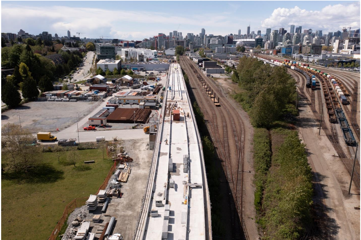
Figure 1: Elevated Guideway: Progressing with the installation of the first sections of track switches at the elevated guideway pocket track.
