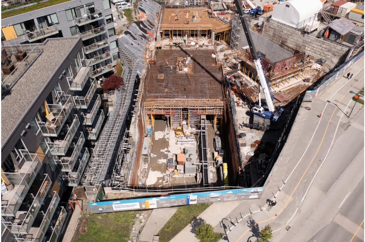
Figure 2: Great Northern Way-Emily Carr Station: Progressing with shoring, rebar and concrete works to construct the concourse level and station roof.
