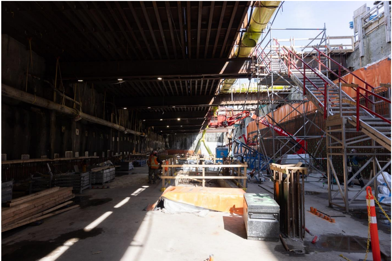
Figure 3: Mount Pleasant Station: Progressing with construction of the concourse-level floor in the station.
