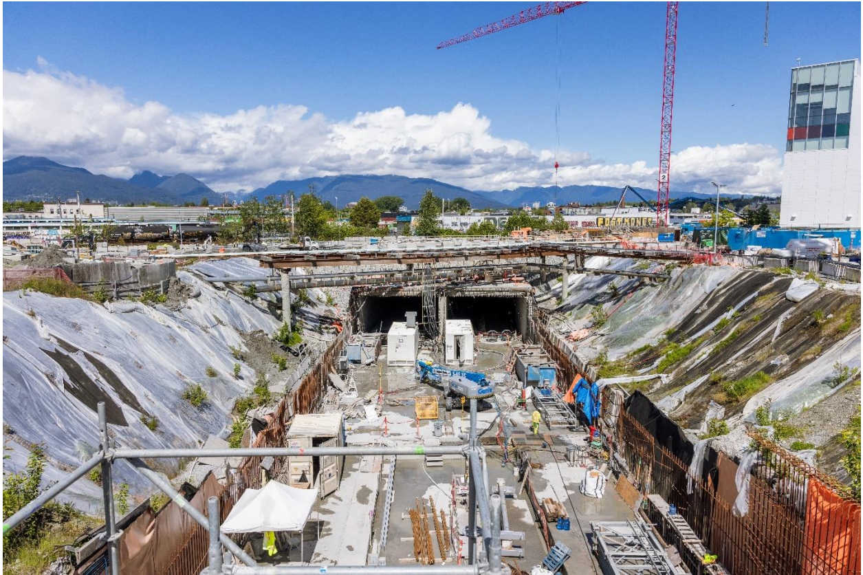
Figure 2: Great Northern Way-Emily Carr Station: View of the transition box looking northeast from the station box area.
