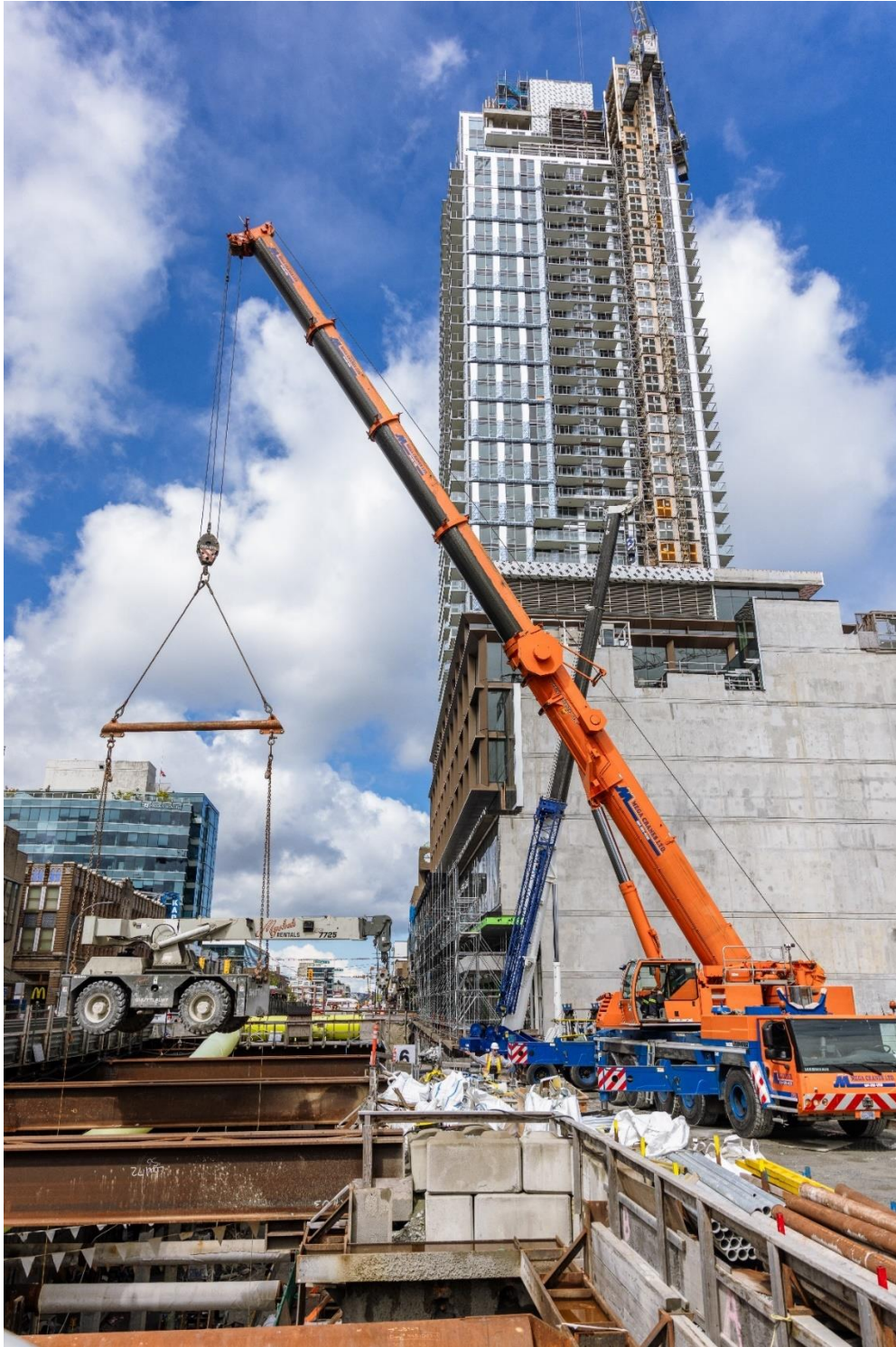
Figure 6: South Granville Station: Removing a small crane from the station box area.
