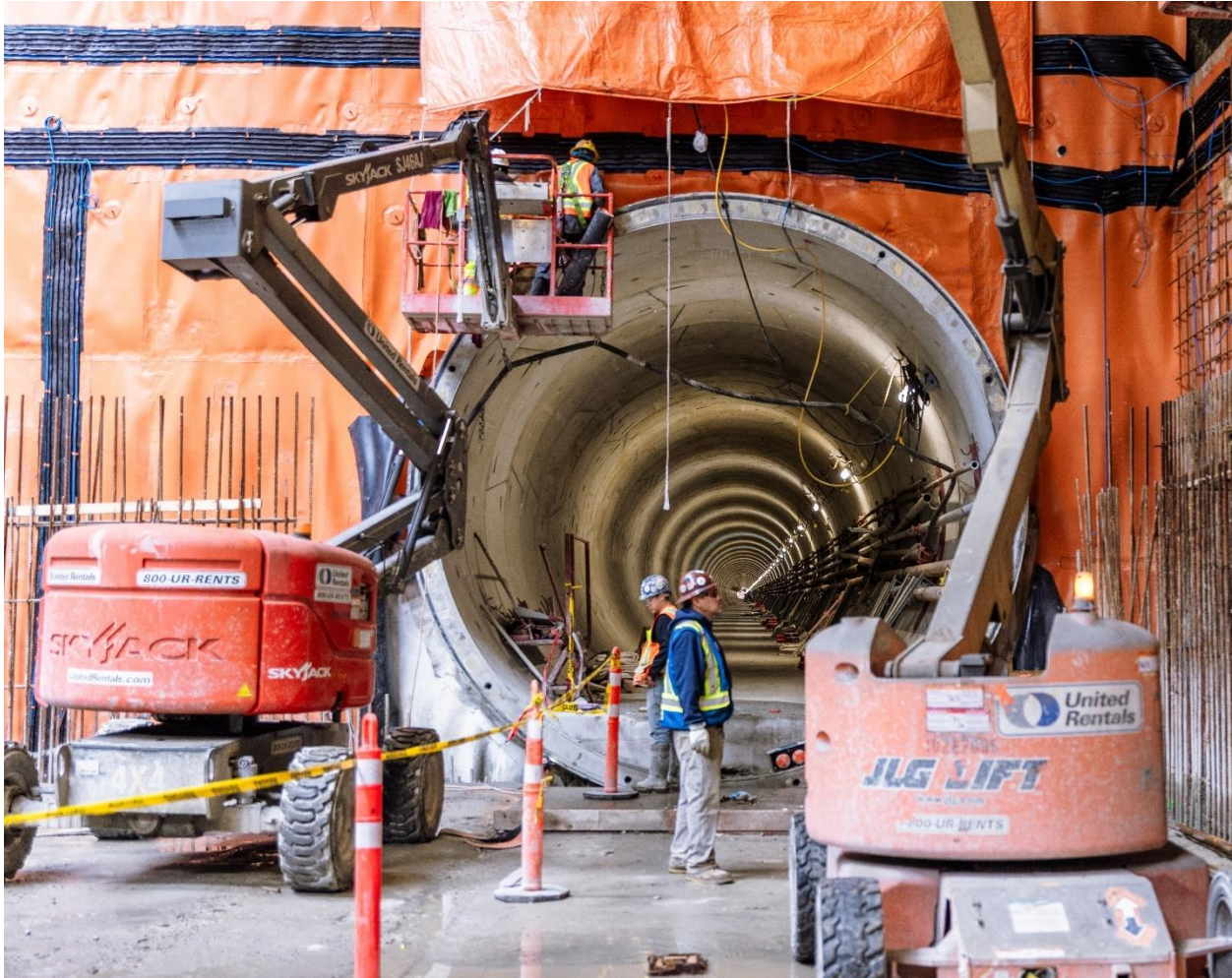
Figure 5: Oak-VGH Station: Ongoing waterproofing in the station box at the west tunnel headwall for the inbound track.
