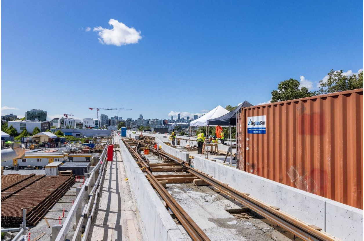
Figure 1: Elevated Guideway: Continuing with the installation of the track switches at the elevated guideway pocket track.
