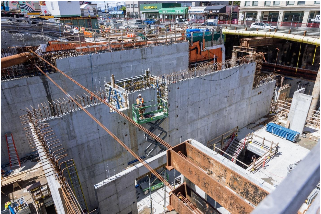
Figure 3: Mount Pleasant Station: Progressing with construction of the headhouse walls for the concourse level.
