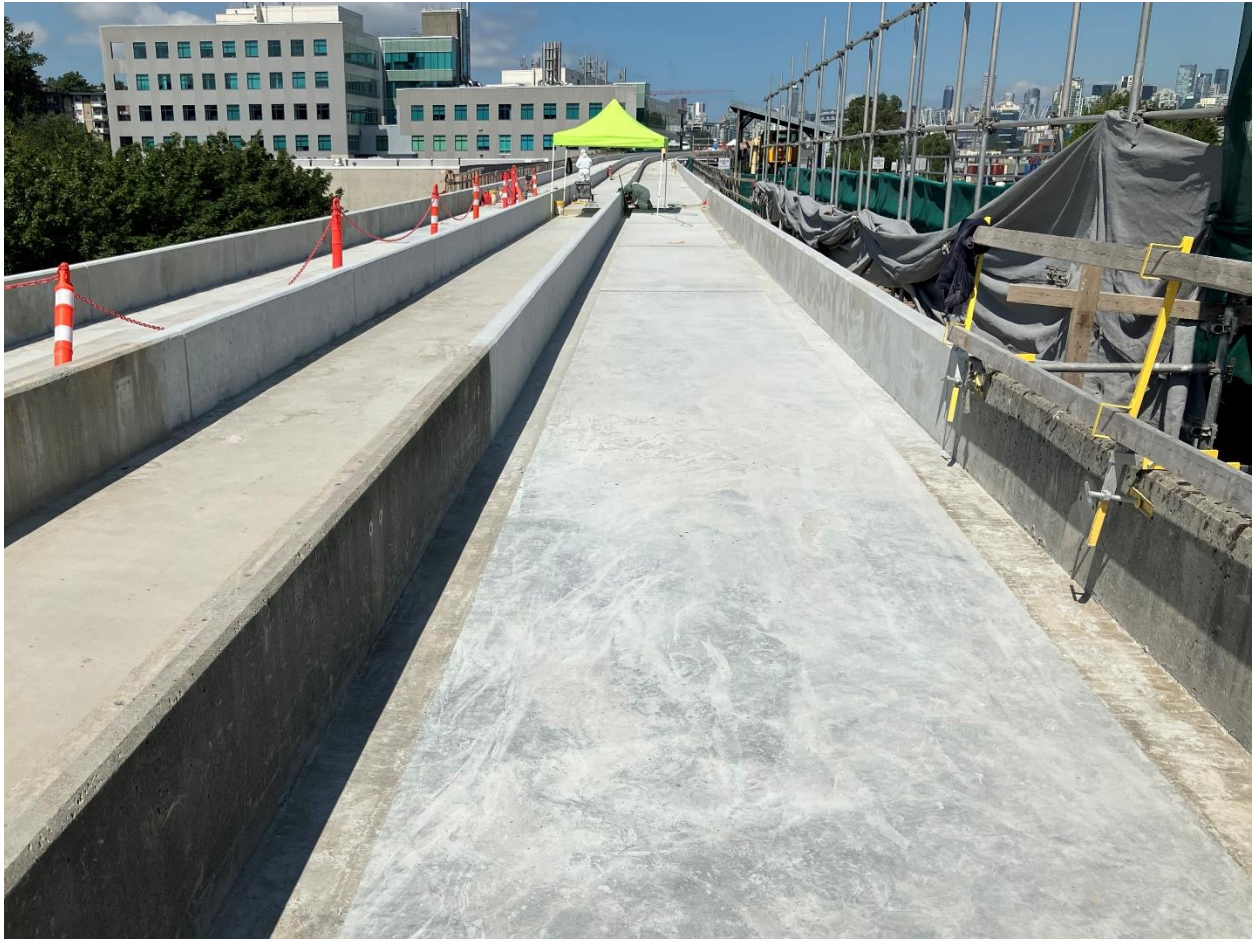
Figure 1: Elevated Guideway: Progressing with the connection to the existing elevated guideway at VCC-Clark Station.
