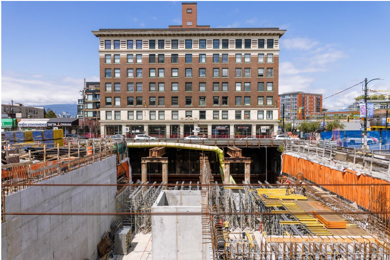
Figure 3: Mount Pleasant Station: Progressing with shoring for the roof slab in the headhouse.
