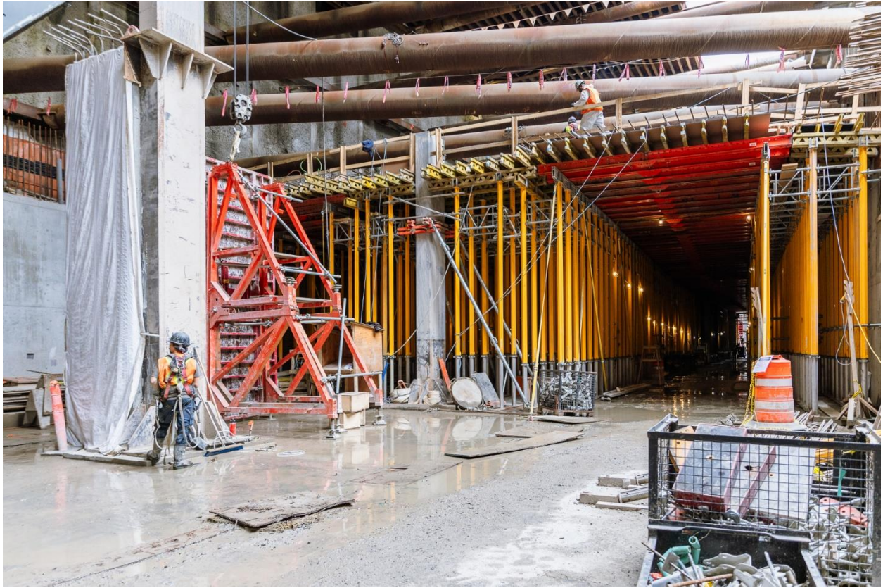
Figure 4: Broadway-City Hall Station: Progressing with construction of the concourse-level floor in the station.
