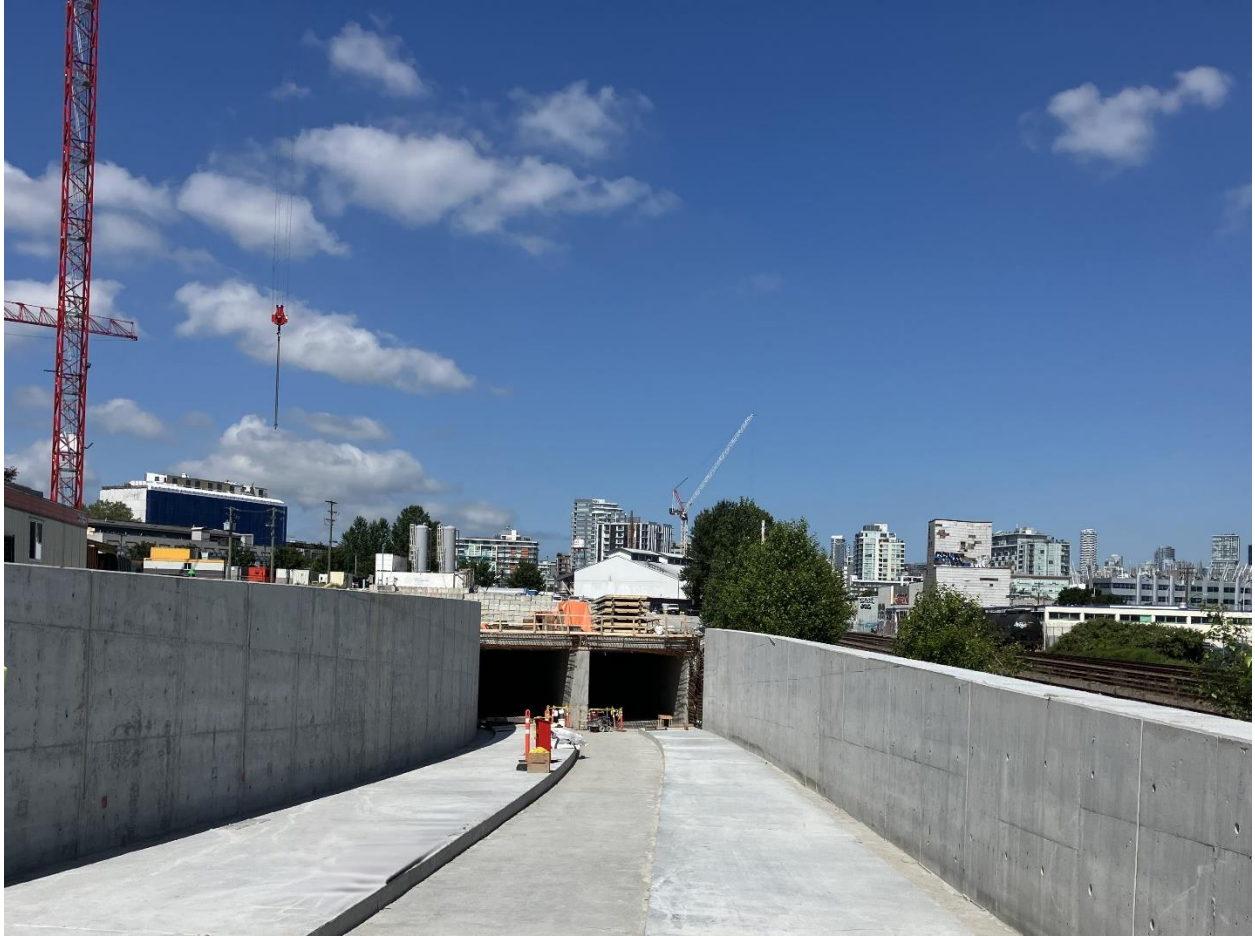
Figure 2: Great Northern Way-Emily Carr Station: Progressing with the walls and track slab installation within the U-Section.
