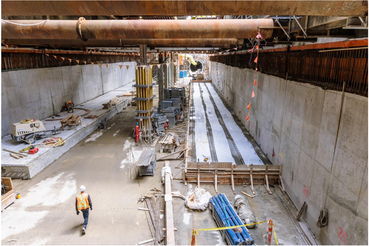
Figure 5: Oak-VGH Station: Progressing with construction of the track slab within the station box.
