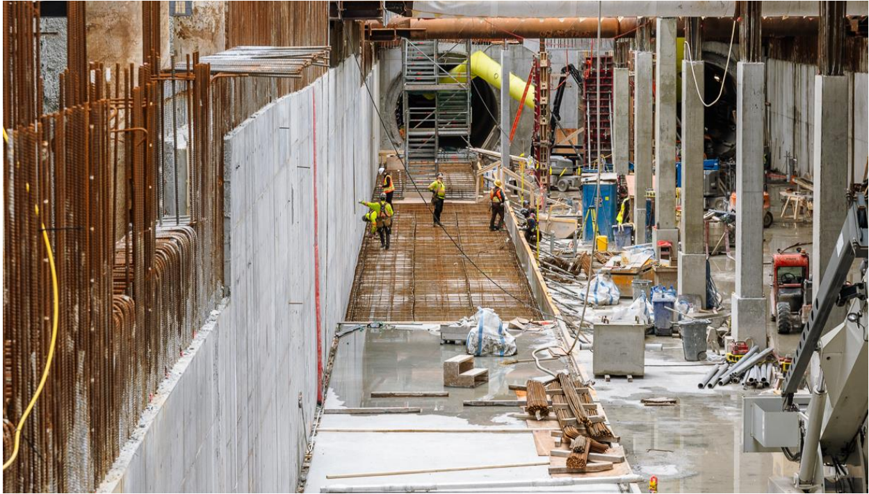
Figure 6: South Granville Station: Progressing with construction of the track slab within the station box.
