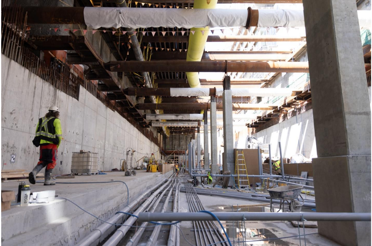
Figure 6: South Granville Station: Progressing with mechanical and electrical conduit installation for the train platform within the station box.
