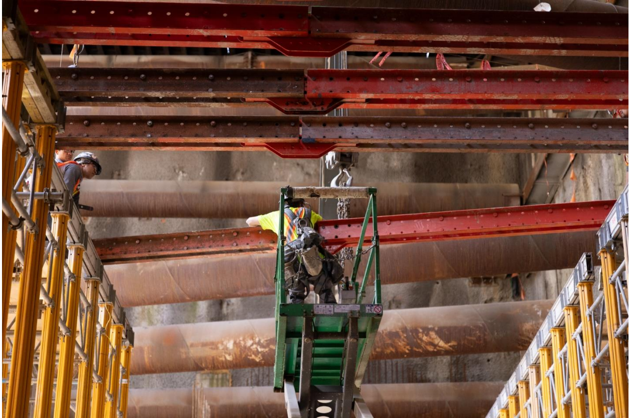
Figure 4: Broadway-City Hall Station: Progressing with work to construct the concourse level within the station box.
