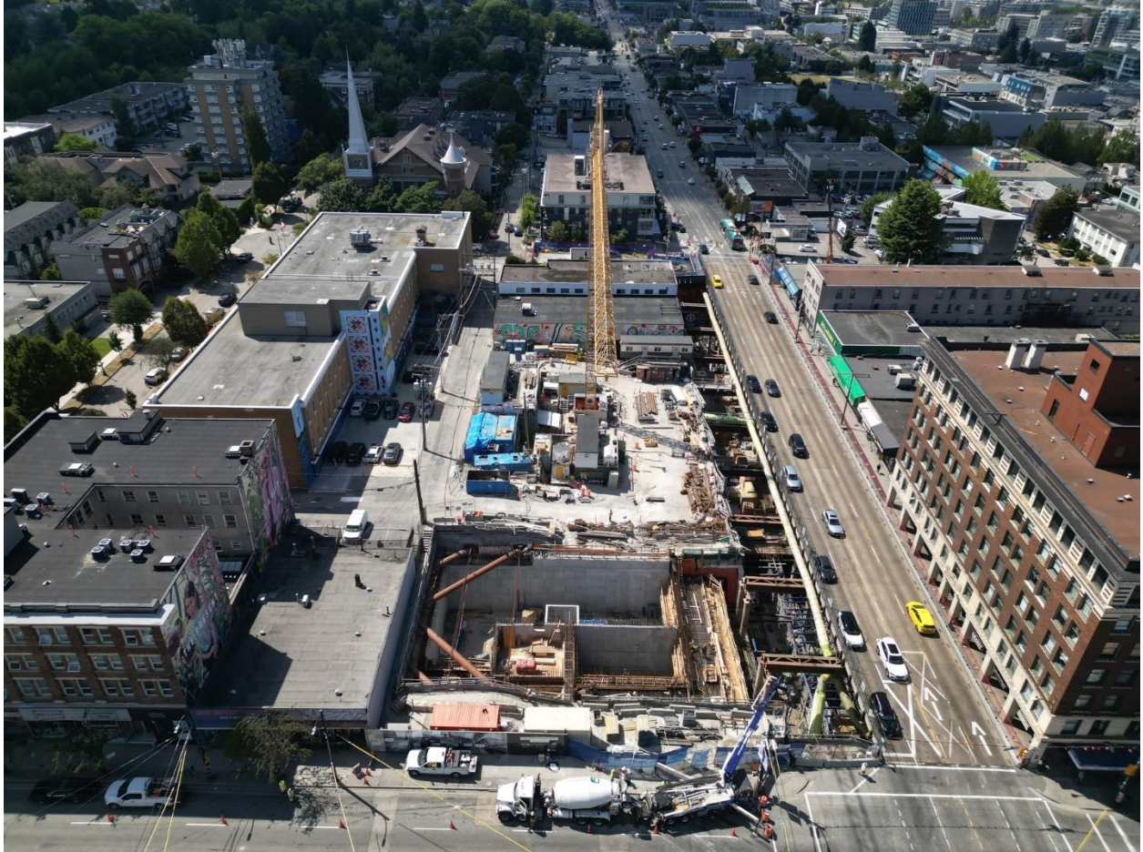
Figure 3: Mount Pleasant Station: Progressing with rebar installation for the roof slab in the headhouse.
