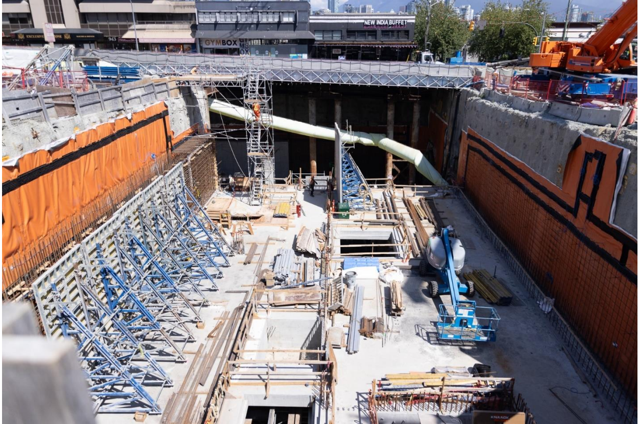
Figure 5: Oak-VGH Station: Progressing with rebar installation and concrete pours for the concourse-level walls in the headhouse.
