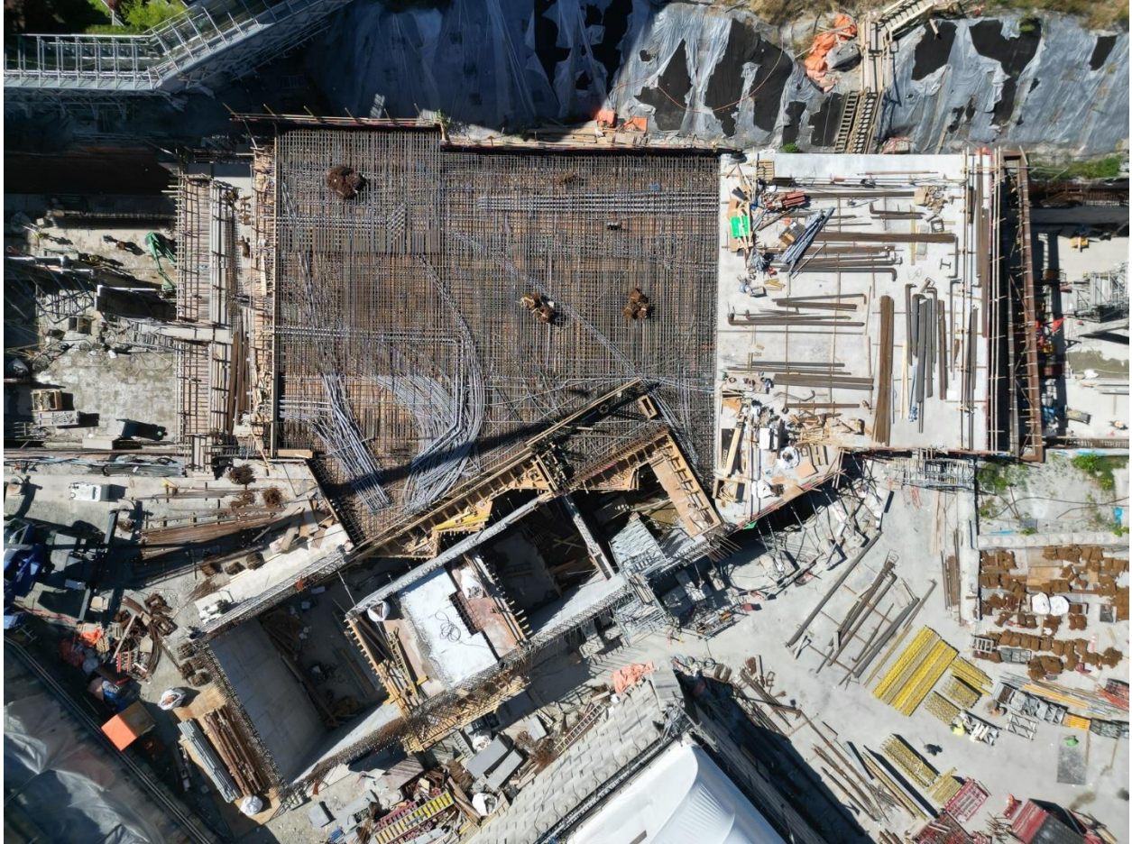
Figure 2: Great Northern Way-Emily Carr Station: Progressing with rebar installation for the second roof slab.
