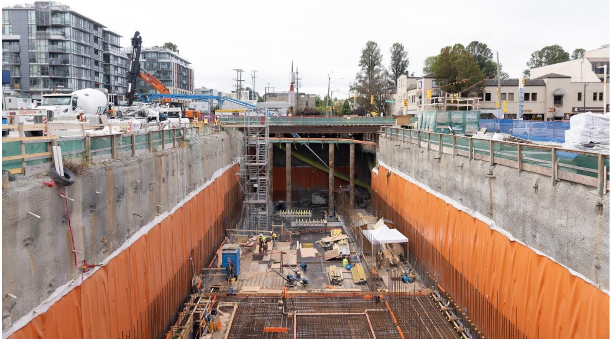
Figure 7: Arbutus Station: Progressing with construction of the concourse-level floor in the headhouse.
