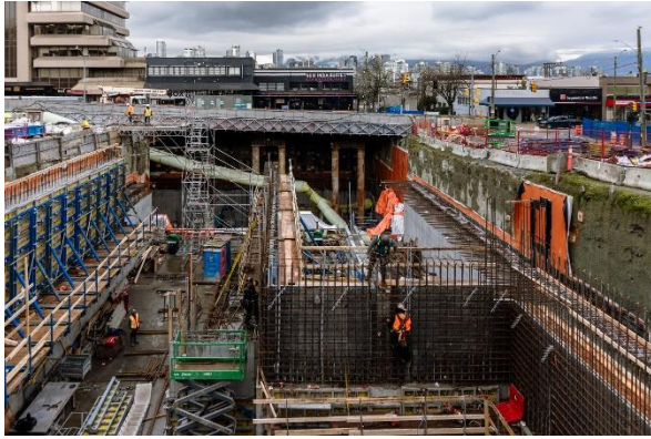
Figure 5: Oak-VGH Station: Progressing with rebar installation for the upper-level interior walls in the headhouse.
