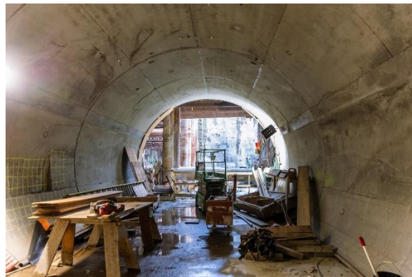
Figure 4: Broadway-City Hall Station: Completing the walls and roof of the tunnelled passenger connection to the Canada Line southbound platform.
