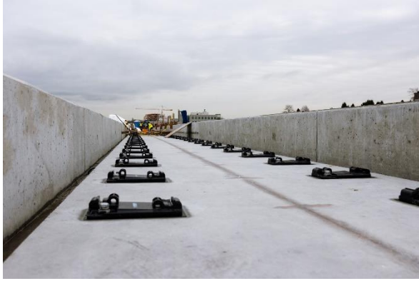
Figure 1: Elevated Guideway: Progressing with coring and installation of fasteners for track installation.
