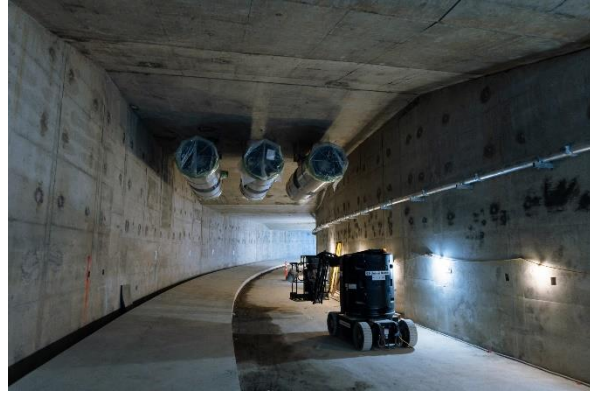
Figure 2: Great Northern Way-Emily Carr Station: Progressing with installation of permanent jet fans in the transition box tunnels.
