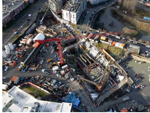
Figure 2: Great Northern Way-Emily Carr Station: Progressing with construction of the station walls and concourse-level floor.
