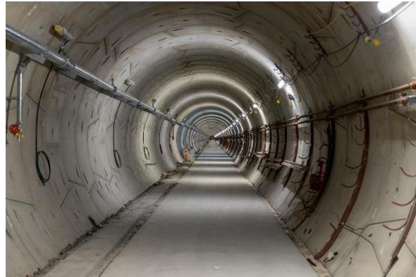
Figure 8: Tunnels: Progressing with construction of the concrete base for the SkyTrain tracks near Oak-VGH Station.
