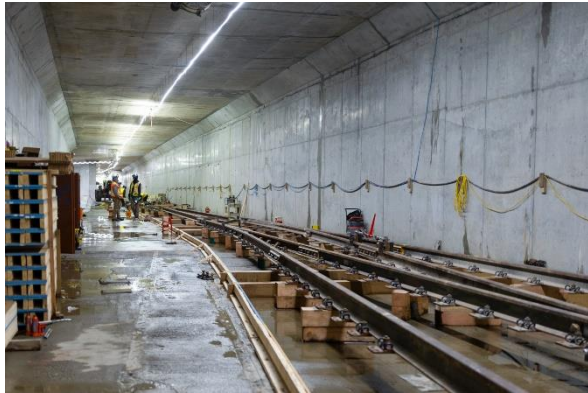
Figure 7: Arbutus Station: Progressing with installation of track switches in the crossover box.
