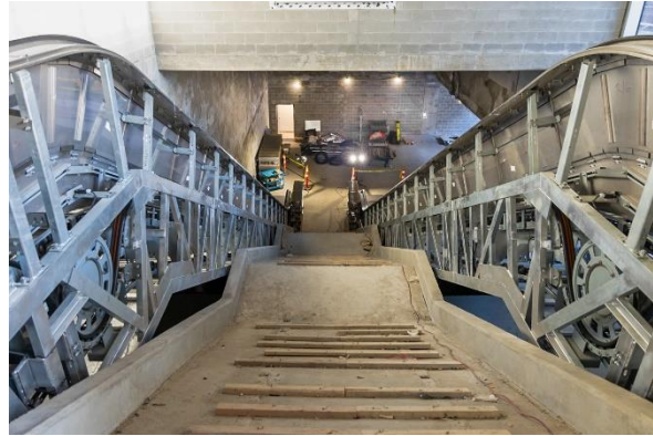
Figure 6: South Granville Station: View from the top of the stairs in the headhouse.
