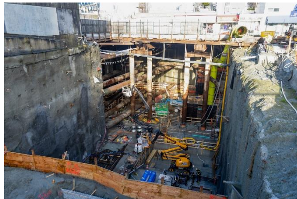
Figure 4: Broadway-City Hall Station: Progressing with the mud slab and waterproofing in the headhouse.
